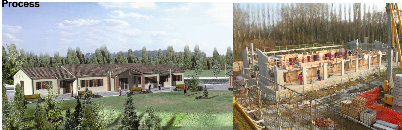
Picture 3 – Class A Training centre and didactic hostel – render and factual realization
